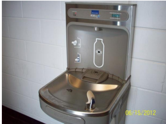
The 1 st installation, Fitzgerald Gymnasium
